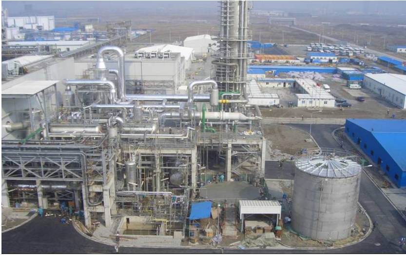
Nitric Acid Plant, Dow + Saudi Aramco
