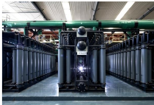
UF membrane racks in Qindao desalination plant
