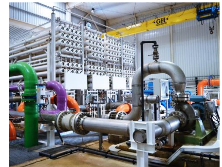
Ghana desalination plant
