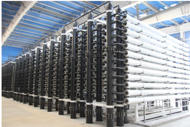
Qinghe tertiary treatment plant
