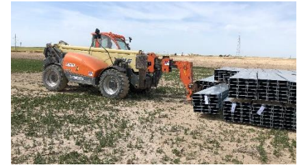
Algibicos (49 MW) Third Party EPC - Spain
