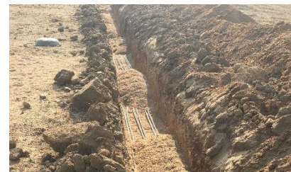
KA2-AFZ (28 MW) Build & Own - India
