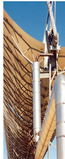
Concentrated Solar Power
