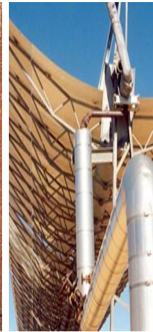
Concentrated Solar Power
