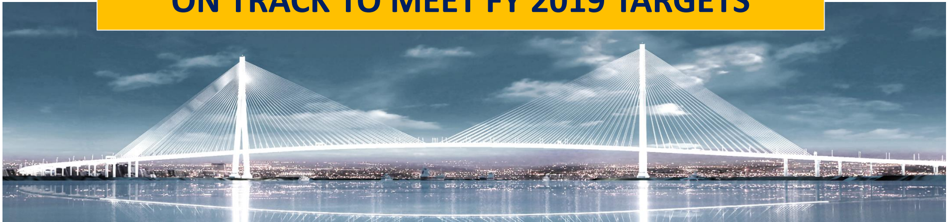
Gordie Howe transnational bridge under construction, linking the cities of Windsor and Detroit, (Canada- USA)
