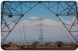
DC and AC transmission lines
