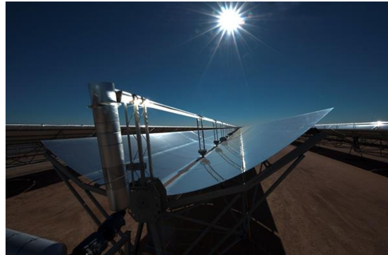
Parabolic Trough: 280 MW Solana
