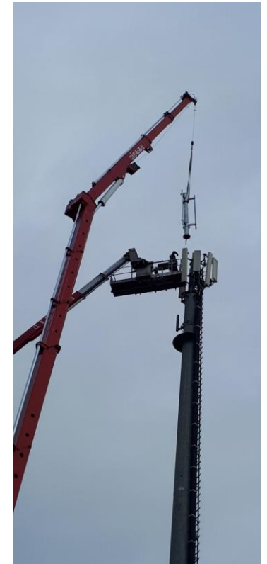
Installing a PoP from the 4 th Italian MNO on a Cellnex site
