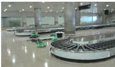
Figure 23. Belts on new trolley park. Gran Canaria Airport
