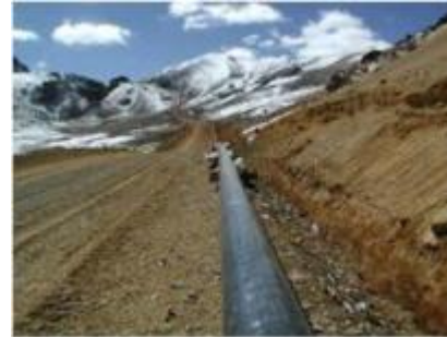
PIPELINE TRANSPORT (NGs & LPGs)
