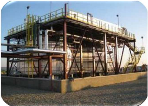
Molten Salts heat storage pilot plant
