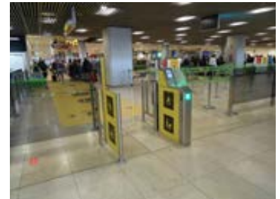
Picture 15. Installation of PRM accesses in the controls of T1 and T4 of Madrid Airport
