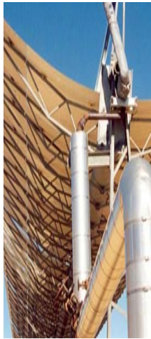
Concentrated Solar Power
