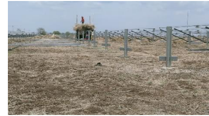
KA2-AFZ (28 MW) Build & Own - India
