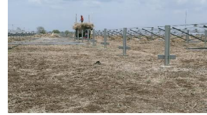
KA2-AFZ (28 MW) Build & Own - India
