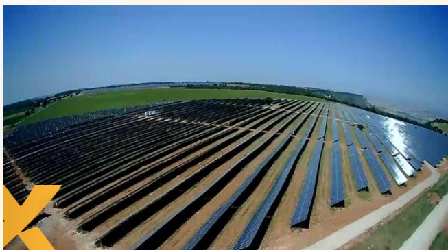
PV Carolinas (Guadalajara) 10 MWp
