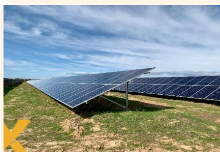
PV Cañamares (Guadalajara) 5 MWp
