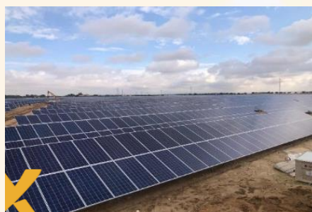
PV Carolinas (Guadalajara) 10 MWp
