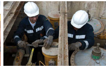
Gas network & service provision – Portugal 1,2M€ - In execution
