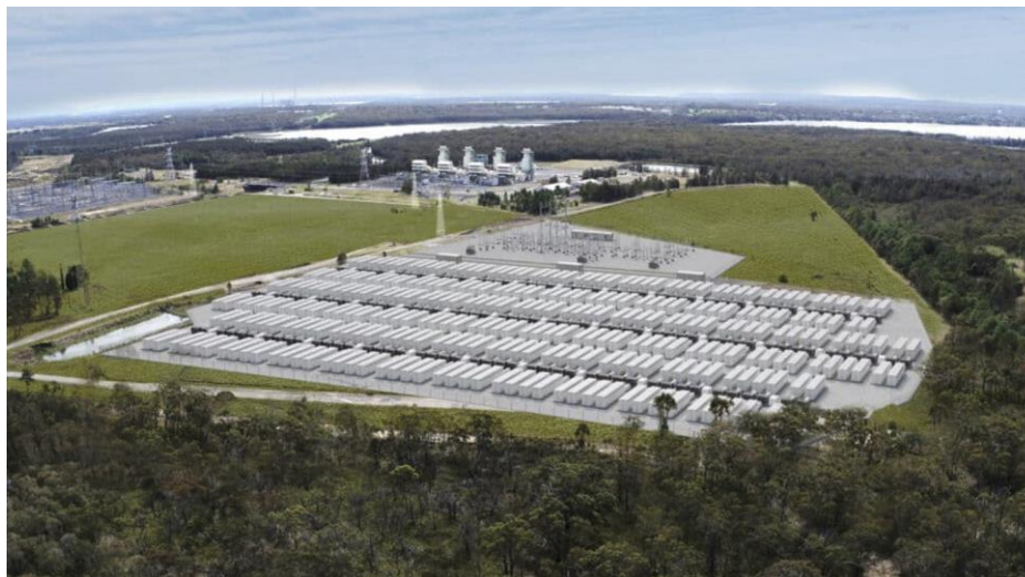
Waratah Super Battery (WSB), Australia
