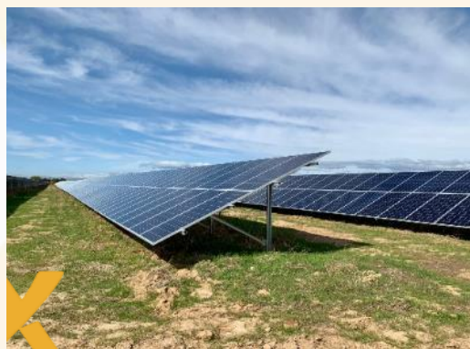
PV Cañamares (Guadalajara) 5 MWp
