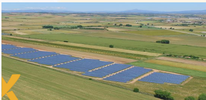
PV Cañamares (Guadalajara) 5 MWp
