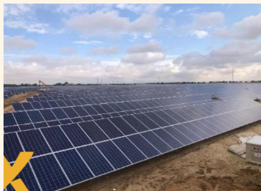
PV Carolinas (Guadalajara) 10 MWp
