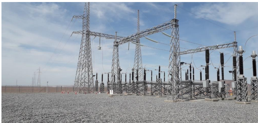
Electrical substation interconnecting Granja to the northern Chilean grid
