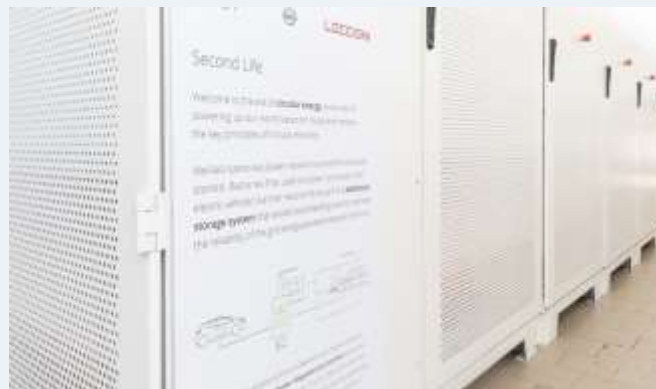
SELF Project in Melilla. Energy storage in second-life batteries.
