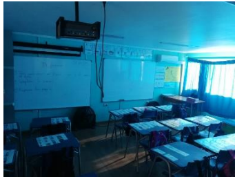
Support for electric installation of Escuela Pintados, Chile
