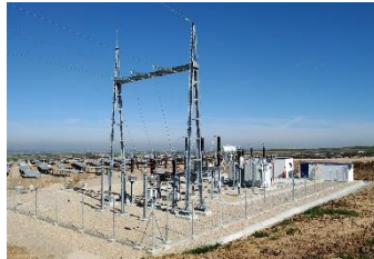
Bargas (50 MW) Third Party EPC - Spain
