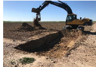
Algibicos (49 MW) Third Party EPC - Spain
