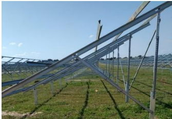
Alvarado (100 MW) Build & Sell - Spain
