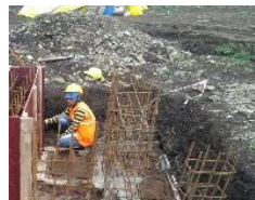
San Antonio 12 MW Build & Sell Chile
