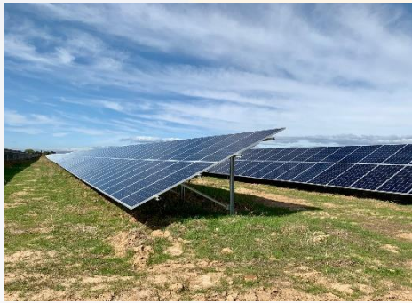
PV Cañamares (Guadalajara) 5 MWp
