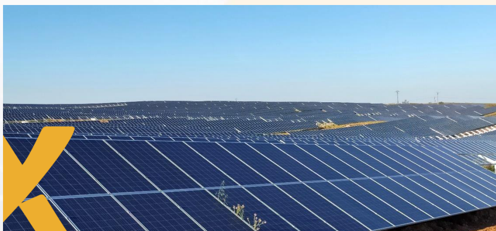
La Zarzuela photovoltaic plant in Toledo
