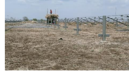
KA2-AFZ (28 MW) Build & Own - India
