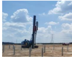
3SP 116 MW Build & Own Malaysia
