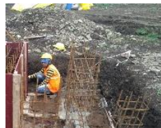
San Antonio 12 MW Build & Sell Chile
