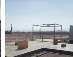
San Marcos 4 MW Build & Own Chile
