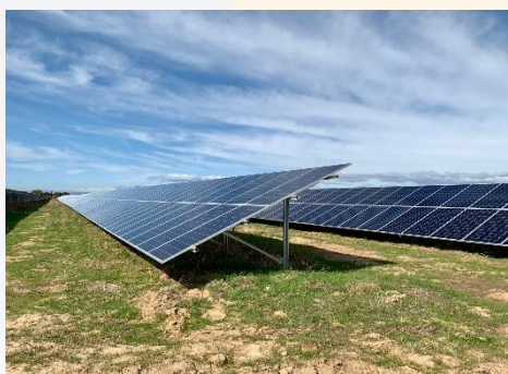
PV Cañamares (Guadalajara) 5 MWp
