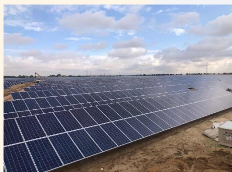
PV Carolinas (Guadalajara) 10 MWp
