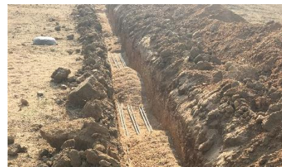
KA2-AFZ (28 MW) Build & Own - India
