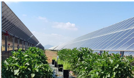
Agrovoltaic project at the Totana photovoltaic plant.
