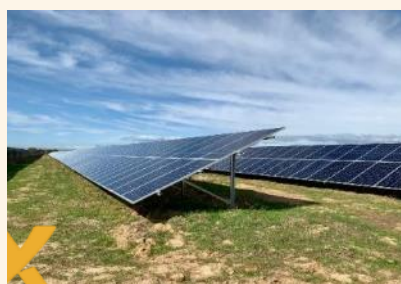
PV Cañamares (Guadalajara) 5 MWp
